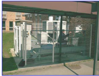
A PlugPower natural gas fuelled CHP unit powers a greenhouse in Nancy, France.
