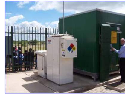
A PlugPower GasCore Fuel System in South Africa provides back-up power for telecommunications.
