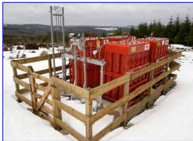
A PlugPower GasCore Fuel System provides power to a telecommunication mast in Scotland, United Kingdom.
